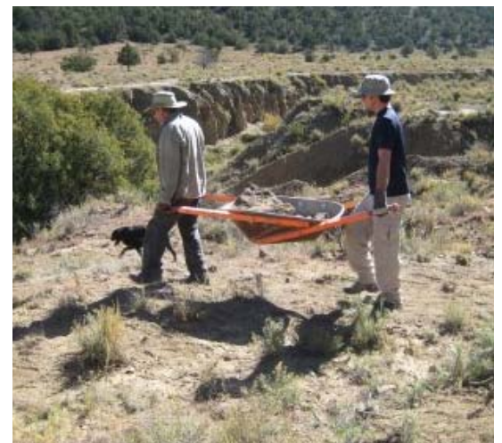
John Canaris (l) and Stephen Bohannon use a rock litter to haul building materials to the edge of the arroyo.
