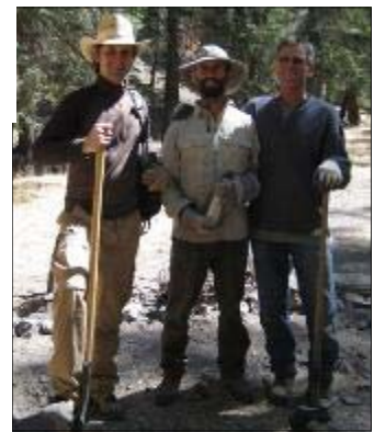
(L to R) Stephen Bohannon, Hamish Thomson, and Gene Tatum pause in their work installing water breaks using logs.
