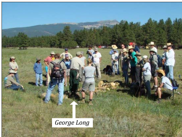
The rock structure crew gathers Saturday morning for instruction on repair procedures from George Long, Wildlife Biologist on Carson National Forest.
