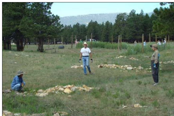
Misako Bradley, Cliff Mendel, and Joyce Mendel (l-r) inspect their repairs to rock structures in the creekbed, while others expand fence enclosures in the background.
