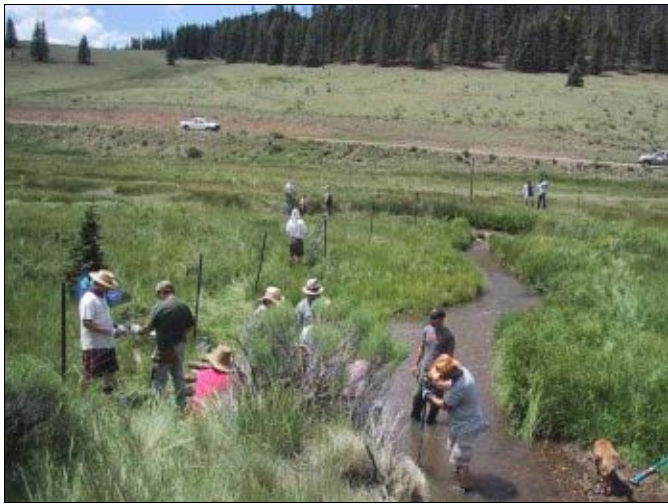
The AWF crew, guided by Bill Zeedyk and ably assisted by the Forest Service's George Long, work on fence exclosures and a large in-stream post vane.
